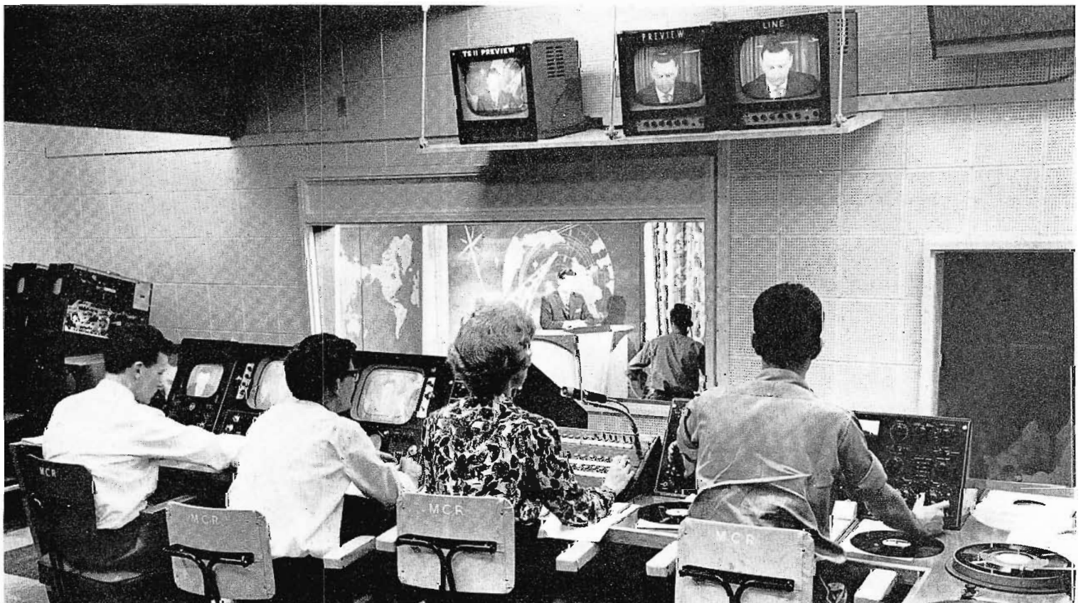
FIG. 12. Master Control serves a three way function as Studio C control room, transmitter control room and master control room. The RCA TS-40 switcher and BC-6B audio console provide flexible programme control facilities.
