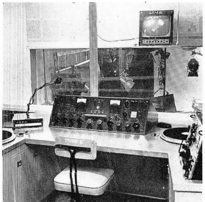
FIG. 10. The BC-6B console in the Studio B audio control room is sometimes supplemented by a four channel auxiliary mixer (not shown).
