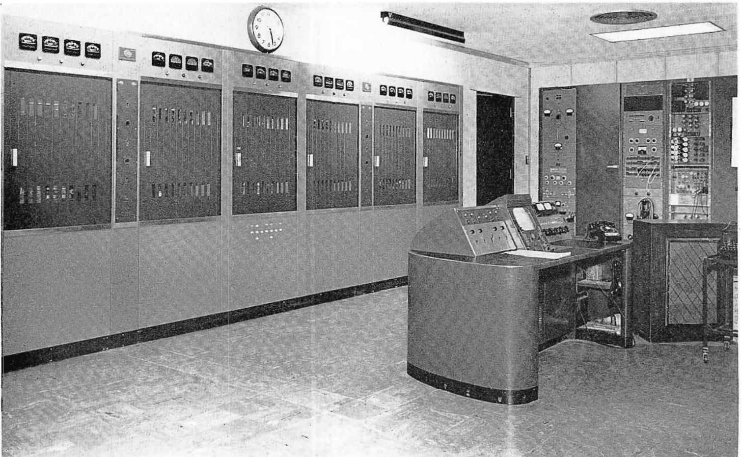
FIG. 21. Type TT-50AH 50 kw TV Transmitter is used by WGN. Together with 12-section superturnstile this gives station maximum of 316,000 watts erp.
