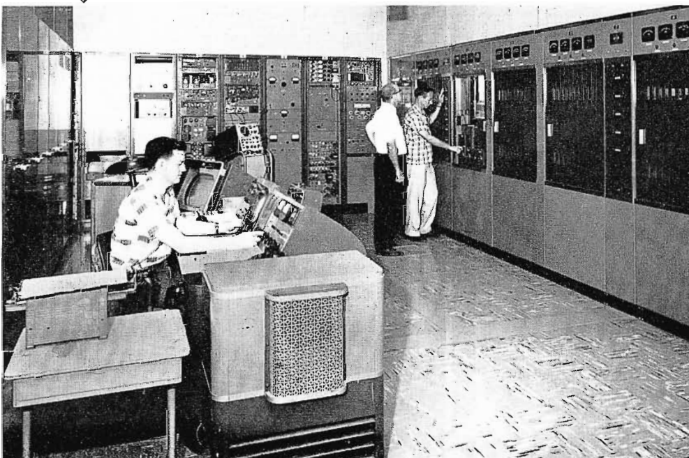
▼ FIG. 5. Television transmitter room showing 25 kw RCA Transmitter (used in conjunction with 12 bay antenna for maximum power).
